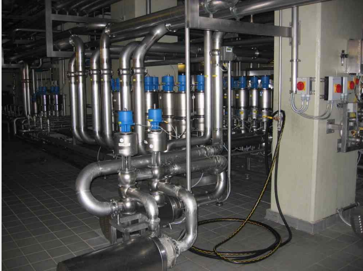
Tank Room - Valves
