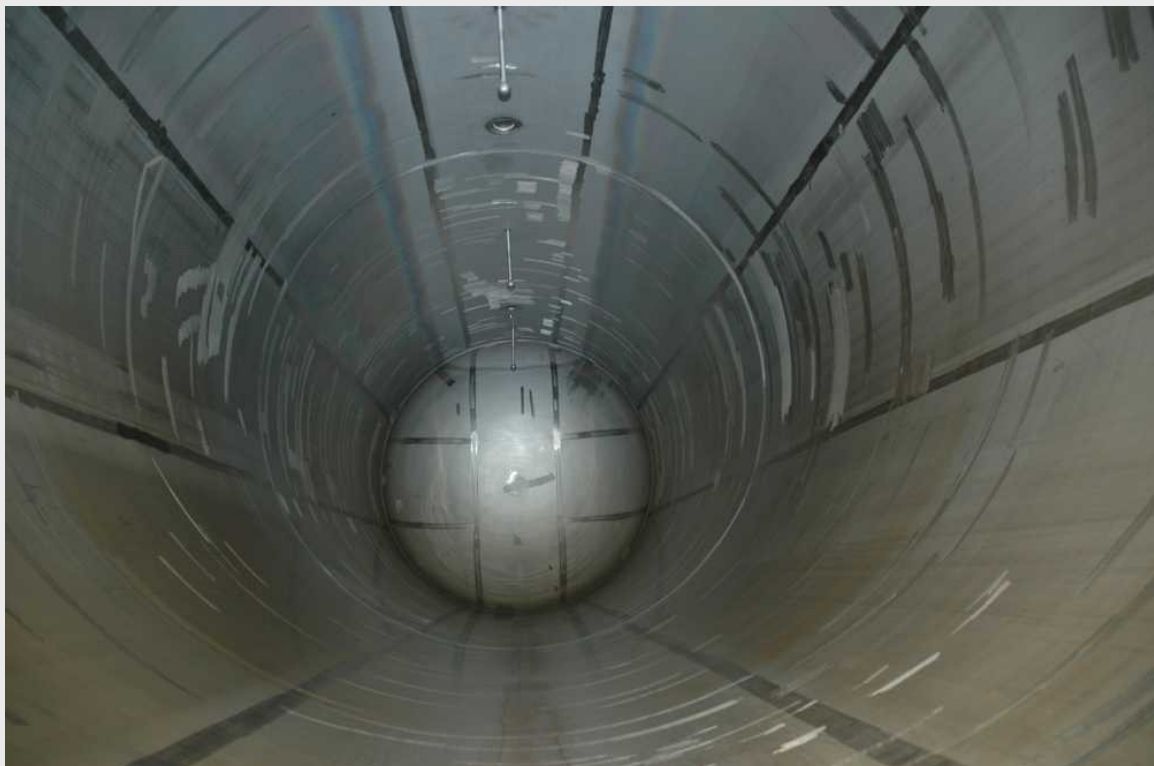
Tanks Horizontal - inside
